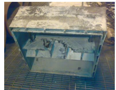
Erosion in Burner tip plates
